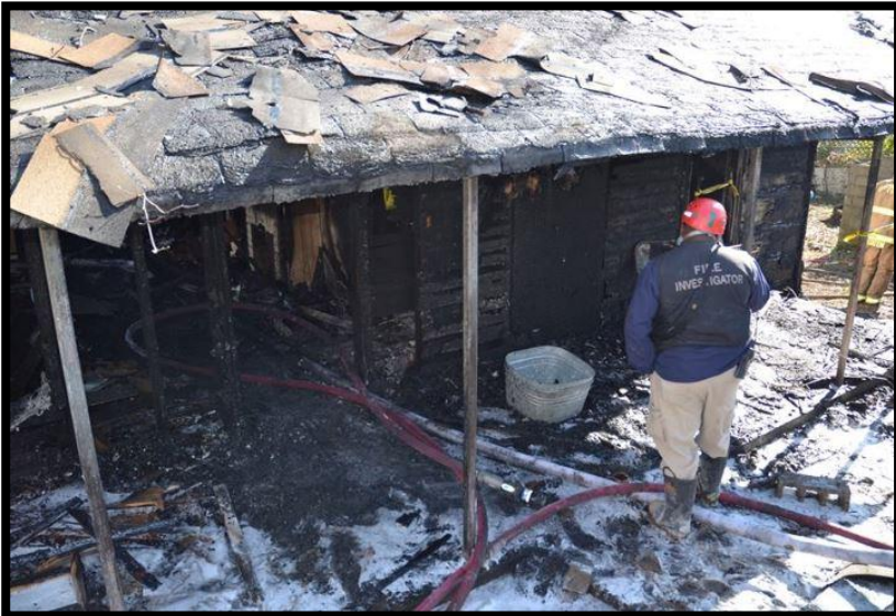
Fire Investigator on scene at recent and tragic Houser Street fire
