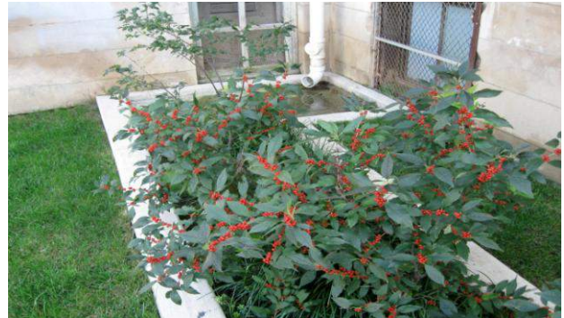
Figure 5.3.11-1. A downspout from an existing building is disconnected to a stormwater planter box.
