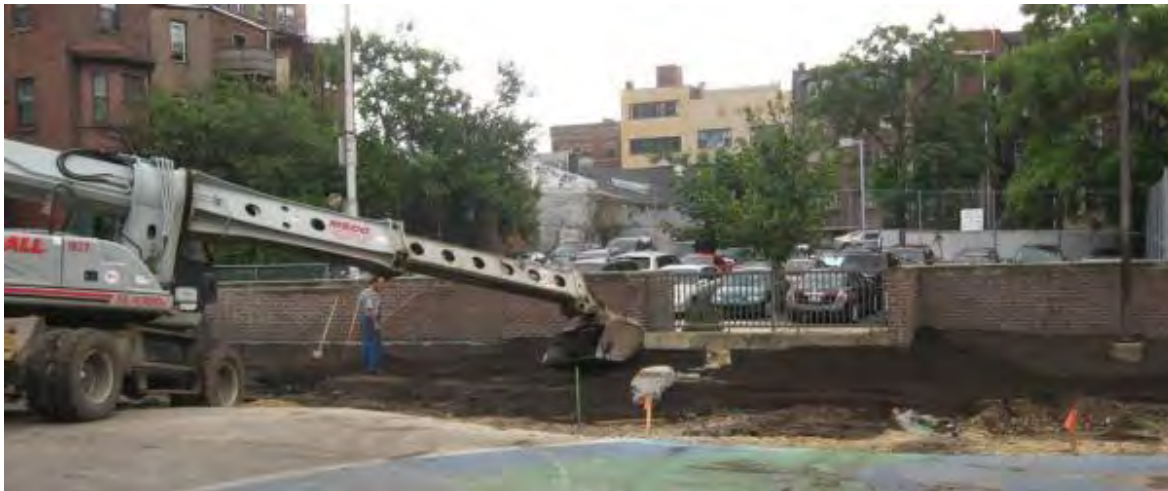
Figure 5.3.4-24. Planting soil is carefully placed in 8-inch lifts to avoid over compaction.
