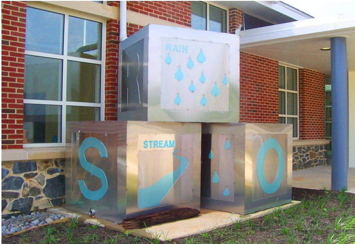
Figure 5.3.9-4. Cisterns can be decorative as well as functional, as is this cistern capturing runoff from a library roof. The cistern, located outside the children’s library, is essentially a rain barrel with a slow-release discharge to the landscape.
