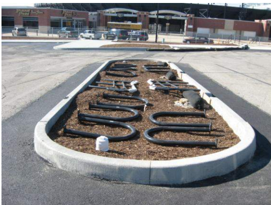
Figure 5.3.11-4. Infiltration planter box within a parking lot, during construction. Water will enter through curb cuts, which are closed during construction. Note that the asphalt around the planter box was milled and repaved, allowing it to drain to the curb cuts following construction.
