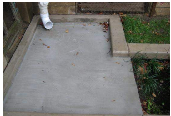
Figure 5.3.11-11. A concrete splash block at a downspout to a flow-through planter box prevents erosive conditions at the soil surface.
