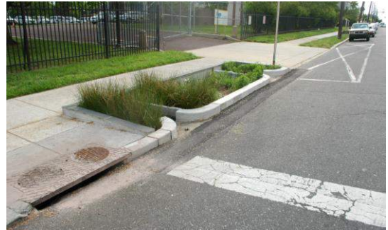
Figure 5.3.11-10. Curb cuts convey street runoff into and out of this streetside planter box. Overflow from the planter box is captured by the downstream storm sewer inlet.
