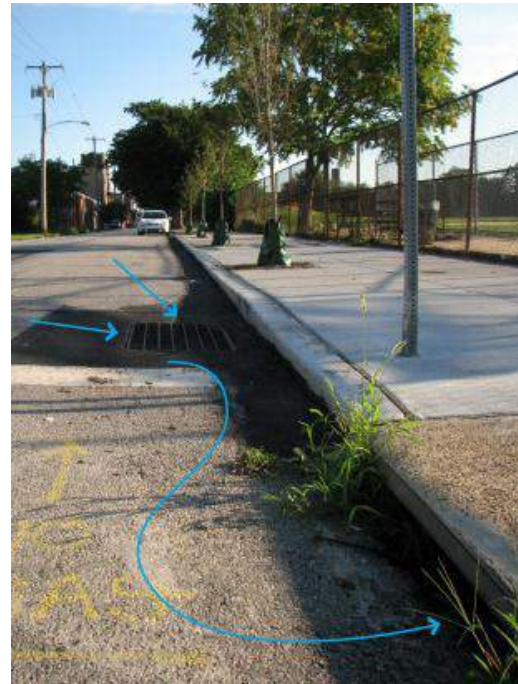
Figure 5.3.3-8. This roadway trench is designed with catch basins to capture and convey runoff into the trench. When the trench is full, flows cannot enter the trench and continue to the next catch basin that conveys the runoff to the larger combined sewer system.
