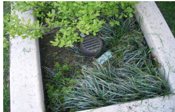
Figure 5.3.11-12. A grated pipe in a stormwater planter box provides overflow to existing storm sewer when ponding above the designed water level occurs on the surface (similar to Figure 5.3.11-2).
