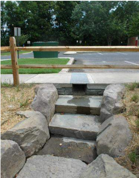
Figure 5.3.5-8. A series of splash blocks prevents erosion on the side of this vegetated swale as runoff enters from a parking lot via a trench drain.
