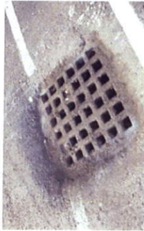
Grease evidence at storm grate. Grease was discharged into stream. Enforcement action was taken.
