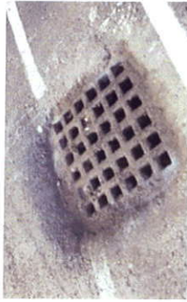
Grease evidence at storm grate. Grease was discharged into stream. Enforcement action was taken.
