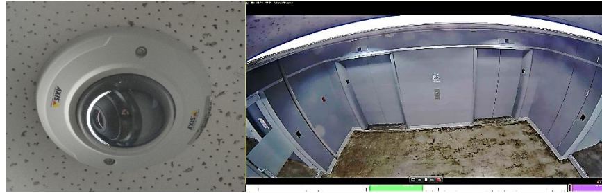
Exhibit 4: Location: Edney Building 3 rd Floor Elevator (Axis M3046-V)
