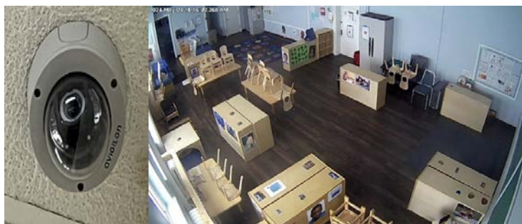
Exhibit 6: Location: Avondale Classroom 103 (Avigilon 3mp H5SL)
