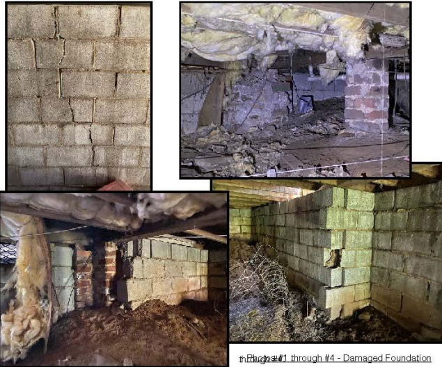
Photos #1 through #4 - Damaged Foundation
