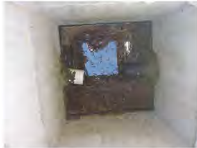
BEFORE MAINTENANCE: Overflow structure basin has sediment and debris (grass clipping) built up in the bottom.
