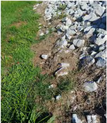
BEFORE MAINTENANCE: Bioretention Pond is full of old grass clippings. Grass clippings have accumulated and clogged the base of the filter dam.
