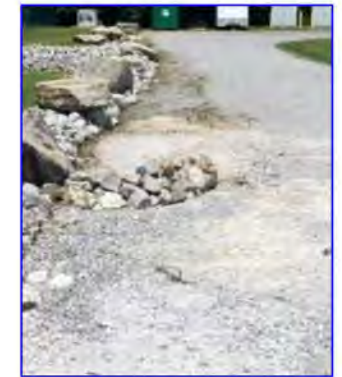
AFTER MAINTENANCE: Removed silt and weeds from washed out area. Replaced gravel, built up the eroded area, and added check dams.
