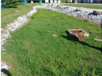
BEFORE MAINTENANCE: Bioretention Pond is full of old grass clippings.
