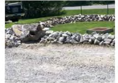
AFTER MAINTENANCE: Removed silt and weeds from washed out area. Replaced gravel, built up the eroded area, and added check dams.
