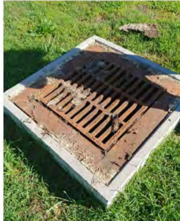
BEFORE MAINTENANCE: Bioretention Pond overflow structure grate has accumulated grass clippings, clogging grate openings.
