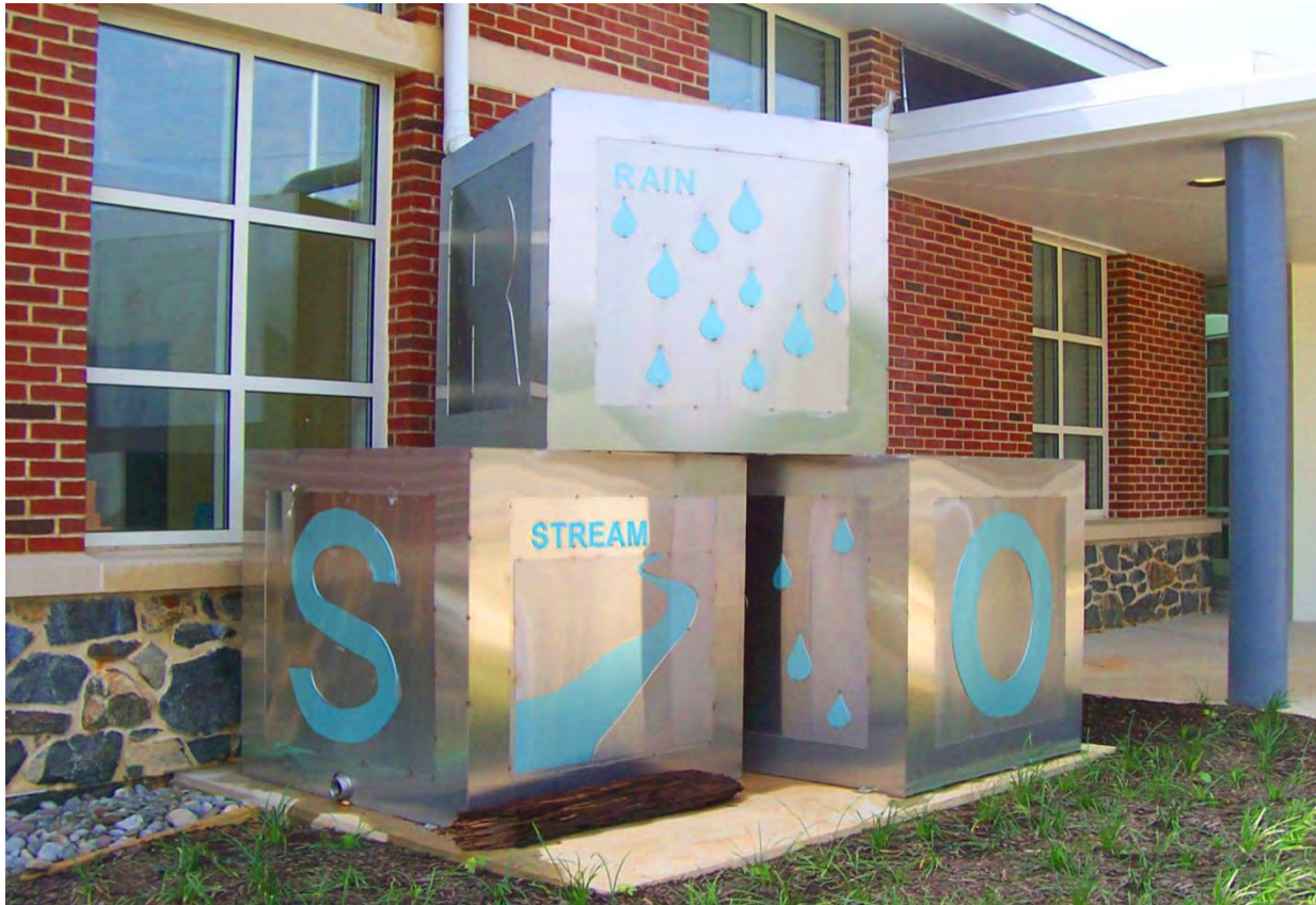
Figure 5.3.9-4. Cisterns can be decorative as well as functional, as is this cistern capturing runoff from a library roof. The cistern, located outside the children’s library, is essentially a rain barrel with a slow-release discharge to the landscape.
