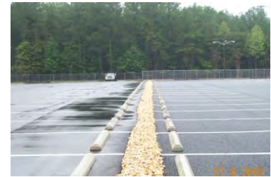
Figure 5.3.1-15. Pervious pavement can be constructed with an unpaved pervious edge treatment. In the event that the pavement is seal coated, clogged, or not functioning, runoff from the pavement can still enter the stormwater bed.
