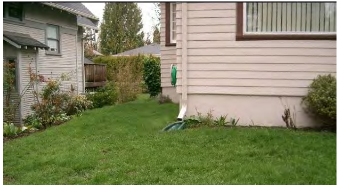
Figure 5.3.10-2. An energy dissipating splash block receives downspout runoff.
