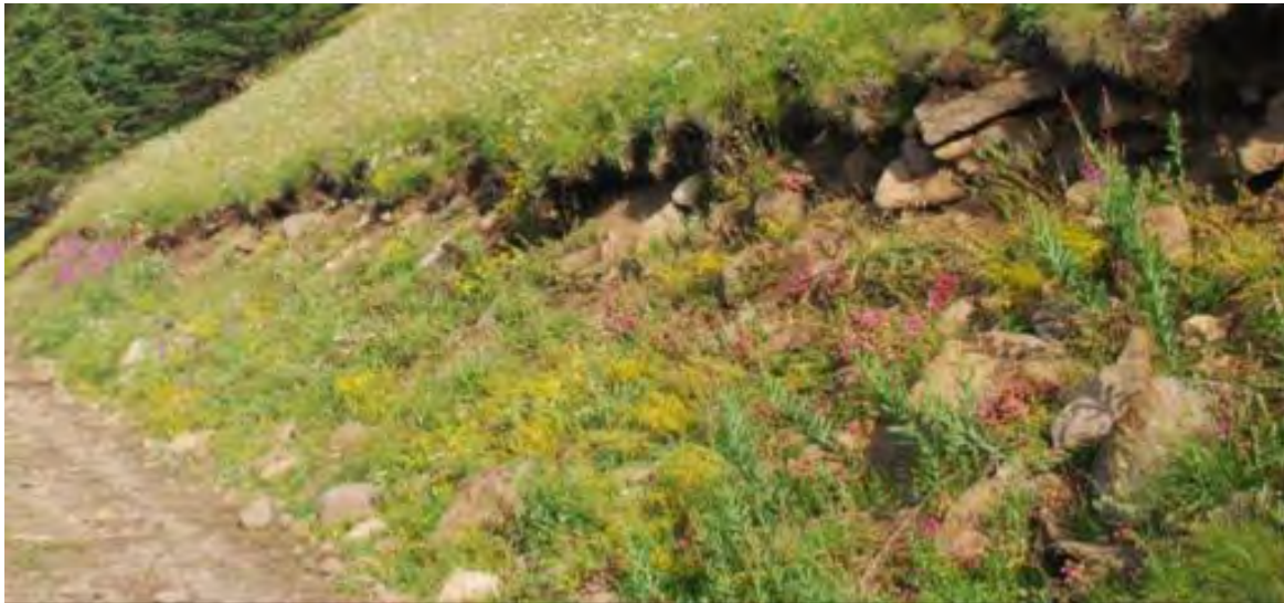
Figure 5.2.4-3. Erosion at steep slope transition.
