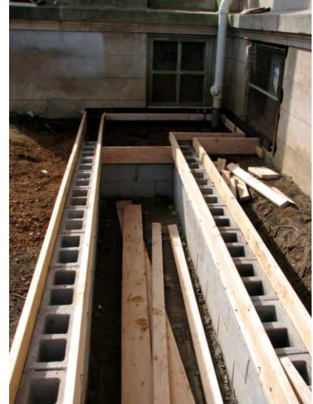
Figure 5.3.11-14. A stormwater planter box during construction. The sidewalls of the planter box are constructed once the final surface grade outside the box is met.
