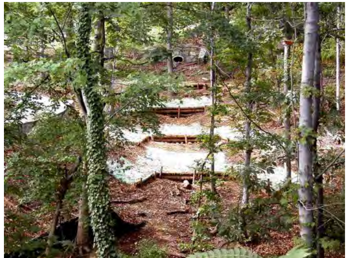
5.2.1.2-9. Check dams below outlet on steep slopes.
