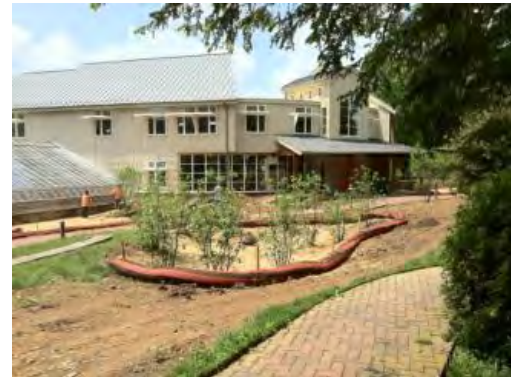
Figure 5.2.2-9. Rain garden during construction using existing stormwater pipes as overflow (note domed riser at center).
