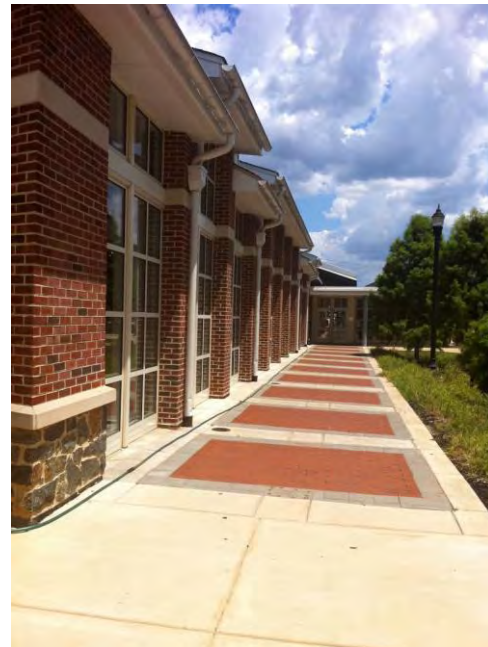
Figure 5.3.4-14. Roof leaders convey runoff below the walkway directly into an adjacent bioretention area. The walk is graded so that runoff sheet flows into the bioretention area. A small filter strip captures any coarse sediment from the walk.
