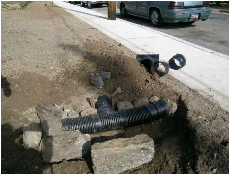
Figures 5.3.5-10. A simple level spreader of perforated pipe can direct flow into a vegetated swale and prevent erosive conditions at the entrance.
