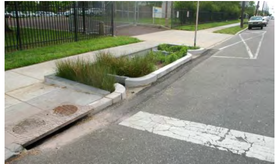
Figure 5.3.11-10. Curb cuts convey street runoff into and out of this streetside planter box. Overflow from the planter box is captured by the downstream storm sewer inlet.
