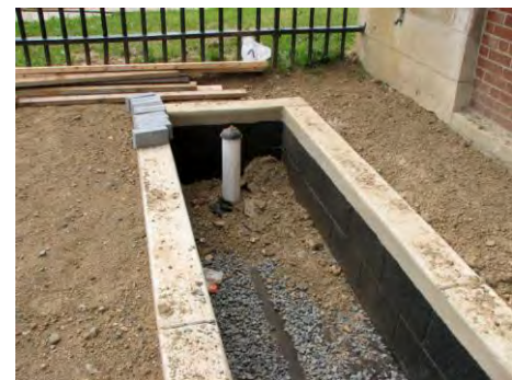
Figure 5.3.11-15. A stormwater planter box that includes a stone bed during construction with geotextile to separate the soil and stone.
