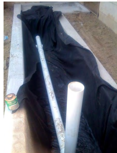
Figure 5.3.11-13. A waterproof liner is placed in the stormwater planter box to protect the adjacent building.
