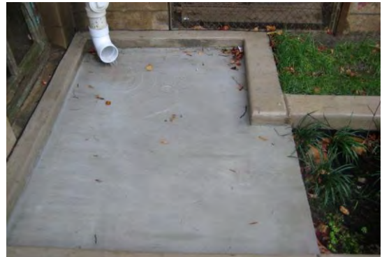
Figure 5.3.11-11. A concrete splash block at a downspout to a flow-through planter box prevents erosive conditions at the soil surface.
