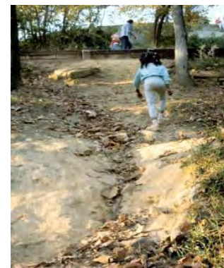
5.2.1.2-4. Gully created by pedestrian cut-through.
