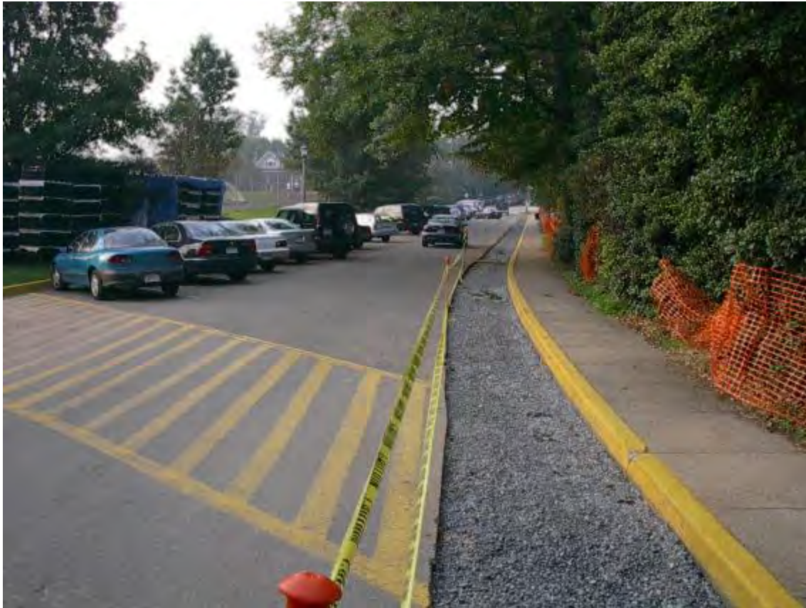
Figures 5.3.3-3a and b. Infiltration trenches were incorporated into an existing storm sewer system within the road at the Washington National Cathedral (Washington, DC). The trench is lined with an impervious liner along the asphalt edge to prevent damage to the roadway subbase from water movement. Overlain by standard asphalt, runoff enters the trench through stormwater inlets.
