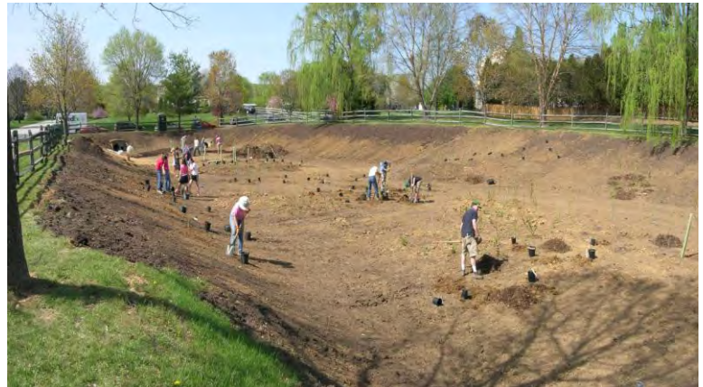
Figure 5.3.13-10. It is important to avoid soil compaction during planting. Retrofit naturalized basins are often good opportunities for volunteer planting efforts if the grading and structural modifications are completed by trained professionals.
