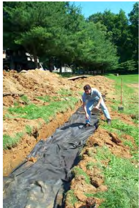
Figure 5.3.3-14. Non-woven geotextile placed between trench and soil prevents movement of soil into trench.
