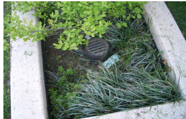
Figure 5.3.11-12. A grated pipe in a stormwater planter box provides overflow to existing storm sewer when ponding above the designed water level occurs on the surface (similar to Figure 5.3.11-2).
